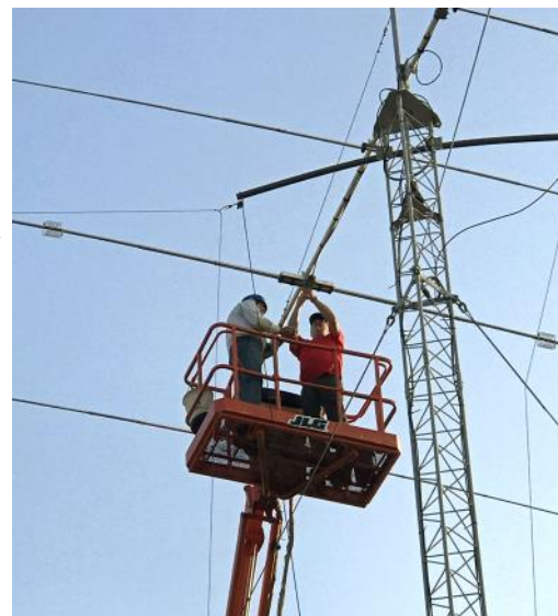
Adjusting the 40m loading coil
