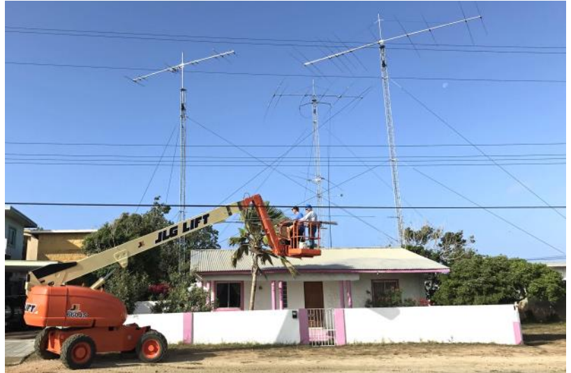
Moving the man lift to access the south tower, right next to the neighbor's house
