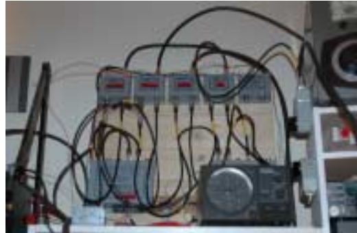
This is a view of WK6I's antenna switching and SteppIR rotation control area.
